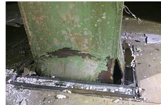
4 days after the earthquake
